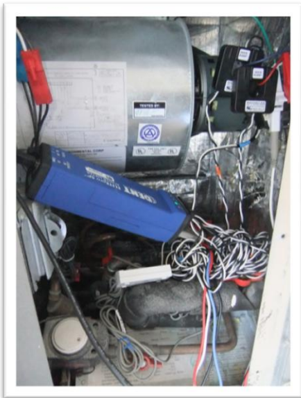
Picture 7: FCU Fan Power Logger and Sensors
