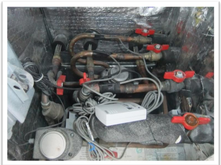
Picture 8: FCU Chilled & Hot Water Temp Logger and Sensors
